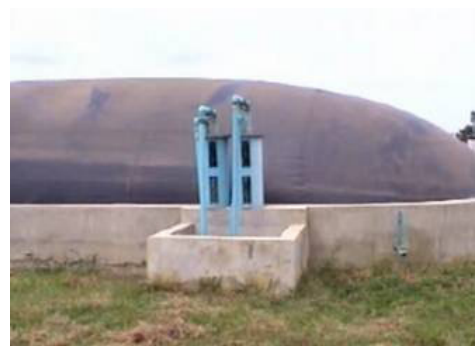
Anerobic Digester Unit
